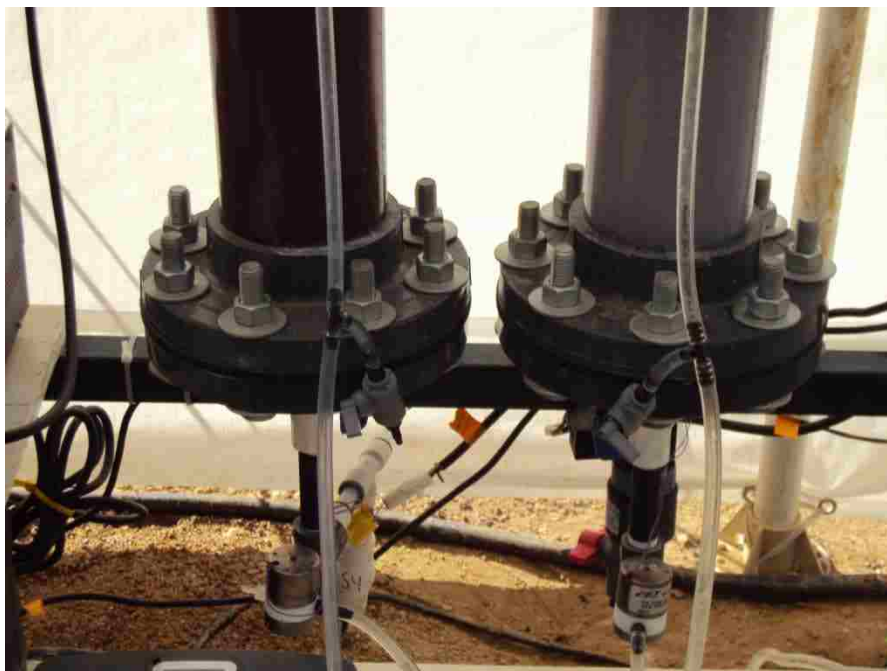
Figure 53: Solenoid Valves at Bottom of Columns
