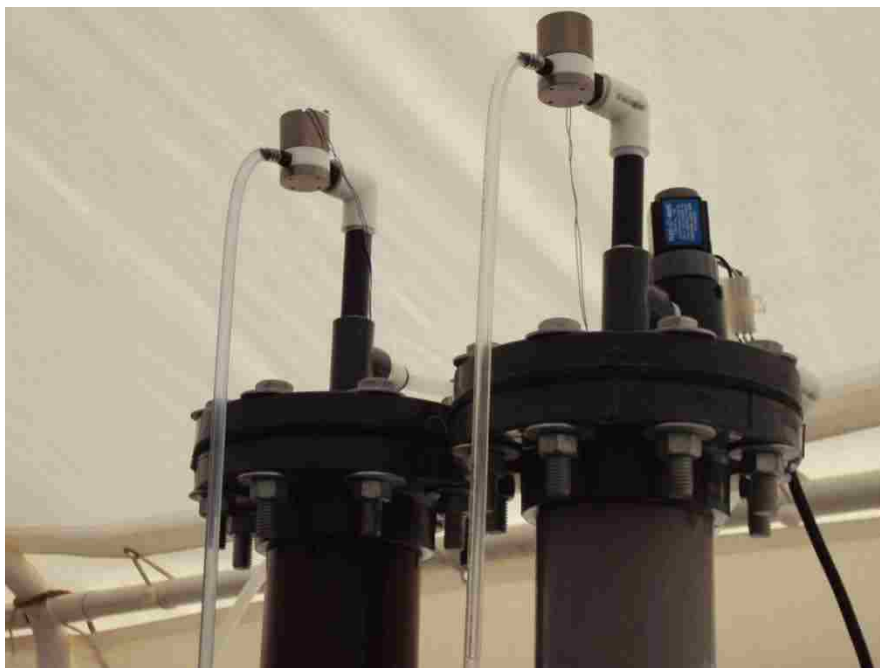
Figure 52: Solenoid Valves at top of Columns
